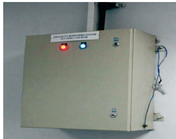
Fig. 8: Main Controller Panel
